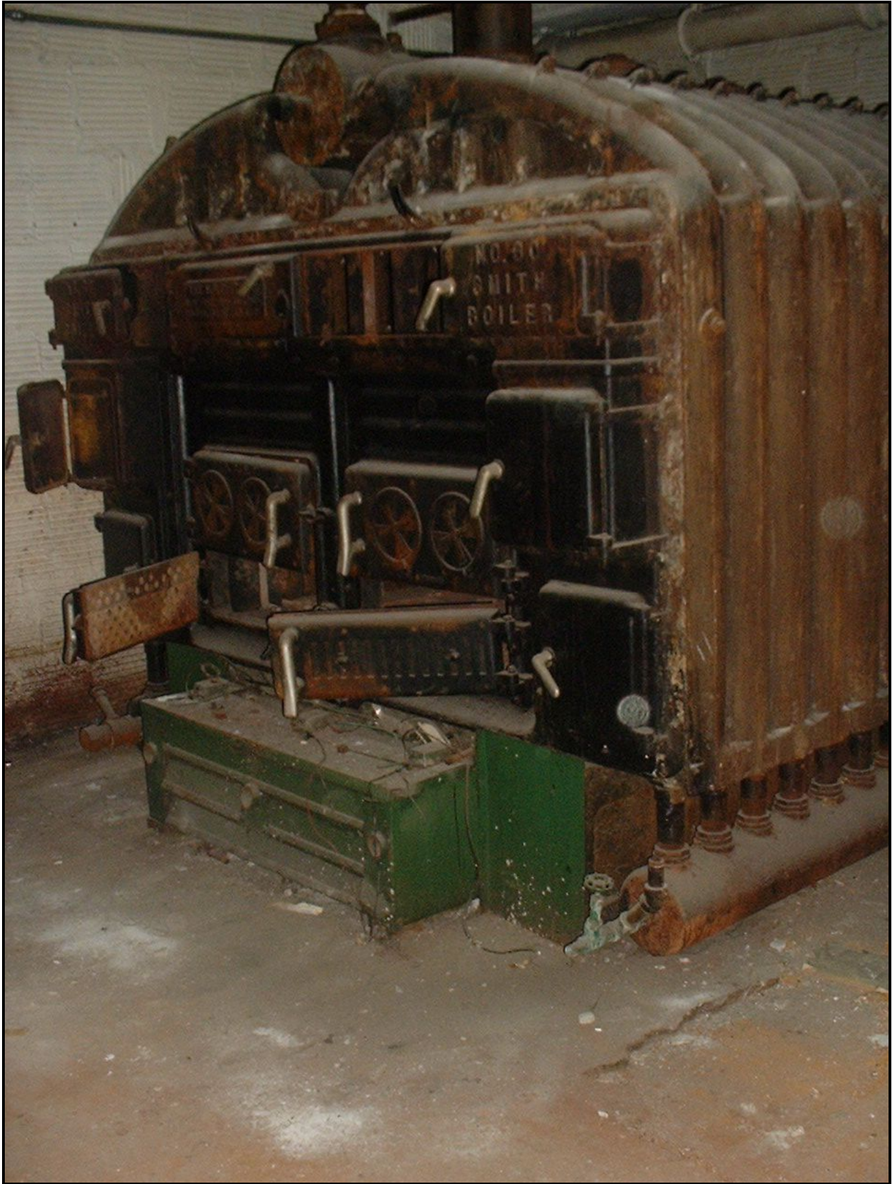
H B SMITH No. 60 BOILER, 196
